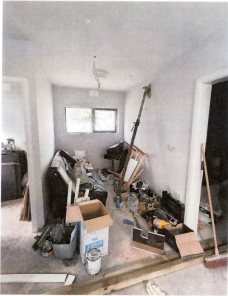
Fig. 7A: The interior of the structure (unchanged from the site visit conducted by the WCC Enforcement Officer)
